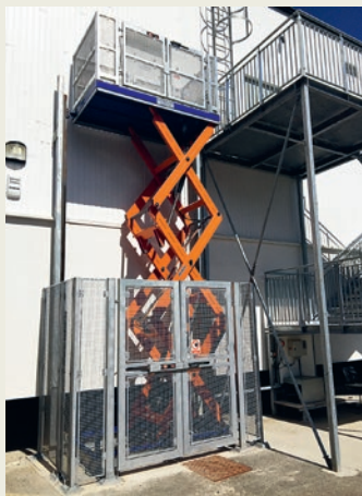
Goods and freight lift
